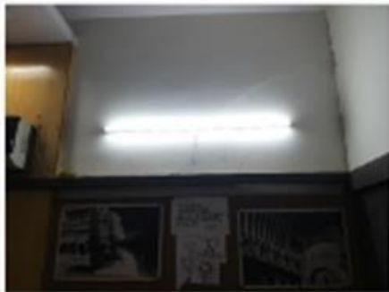
LED lights in staffroom
