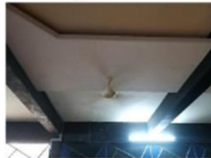
LED lights in Computer room
