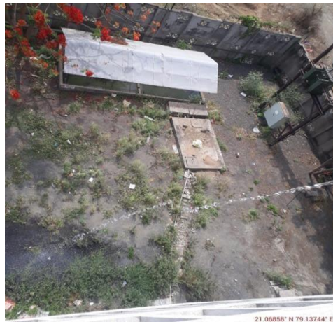
Filter and Storage tank
