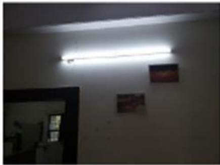
LED lights in Administration
