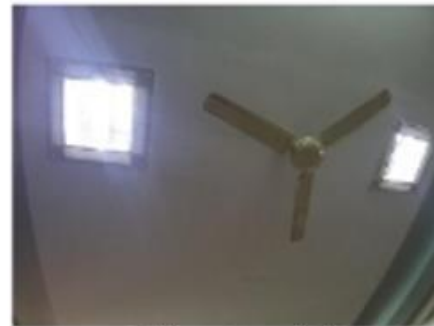
LED lights in Director's Office
