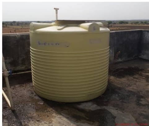
Overhead Storage tank
