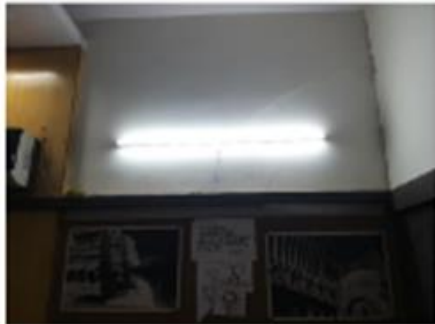
LED lights in staffroom
