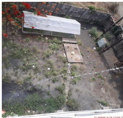
Filter and Storage tank
