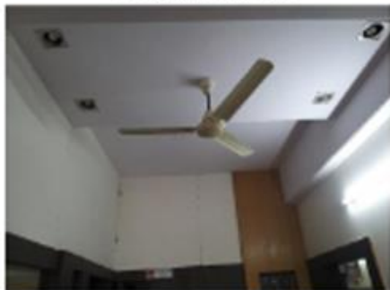
LED lights in Principal's Office
