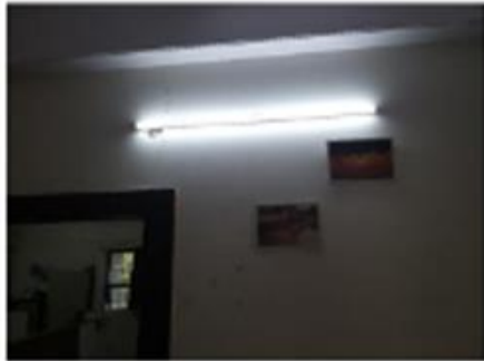
LED lights in Administration
