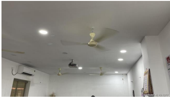
LED lights in conference room
