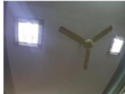
LED lights in Director's Office
