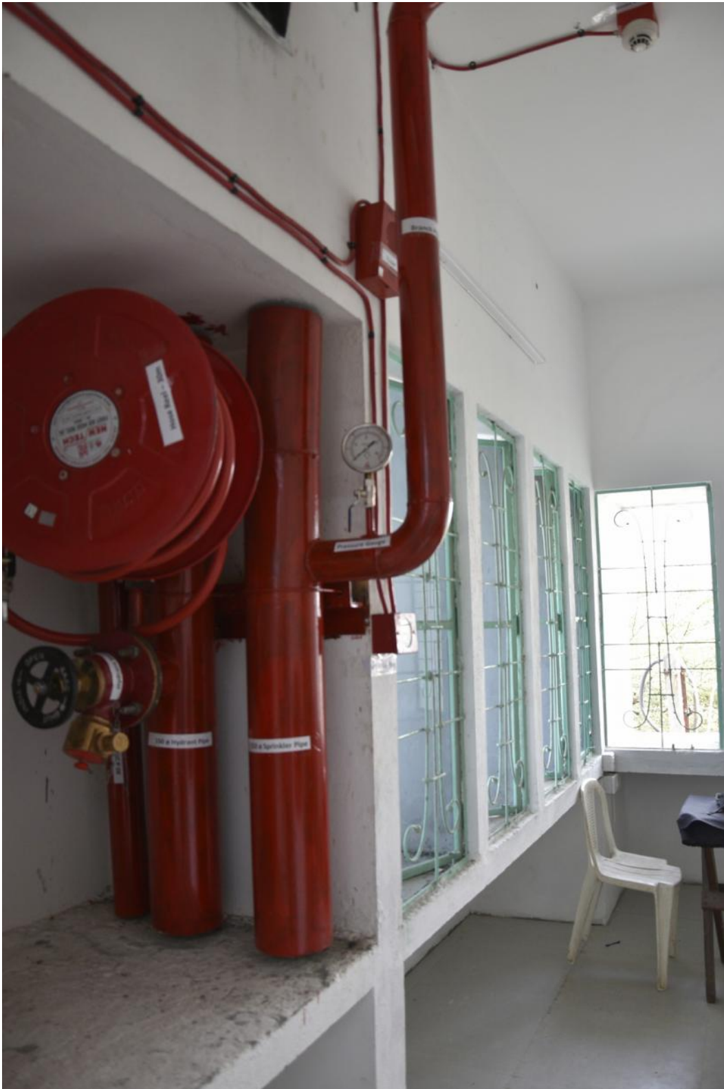
Photograph: Figure III : Building Services
