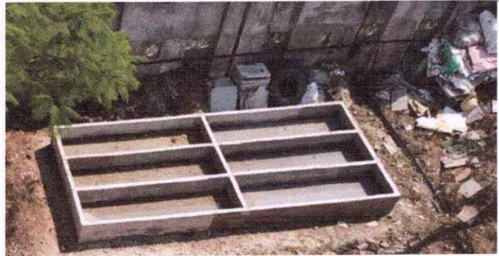
Figure 5 Aerobic treatment tank
