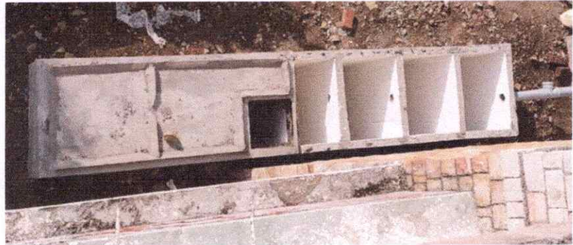
Figure 4 Four chambered anaerobic treatment tank
